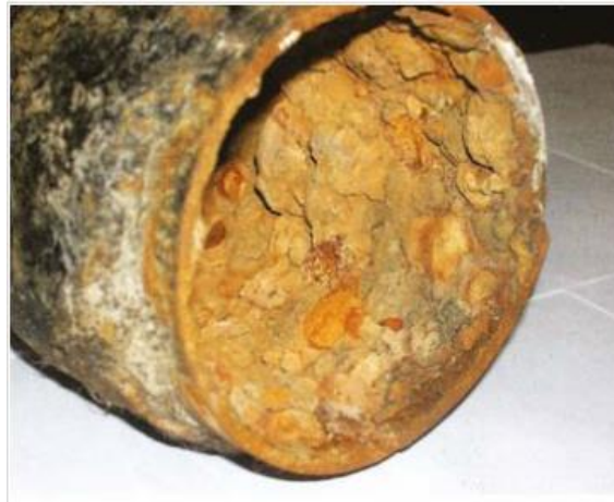
Fig. 16. Typical pipeline failure of fire suppression system - corrosion (Rybar, 2016)
