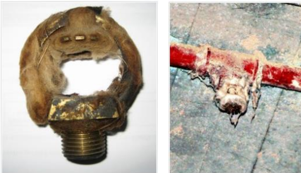
Fig. 15. Typical fault of sprinkler heads (Rybar, 2014)
