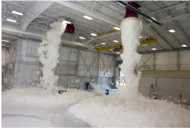
Fig. 3. Example of a hangar fire suppression system in action (Global Aerospace Aviation Insurance, 2021)
